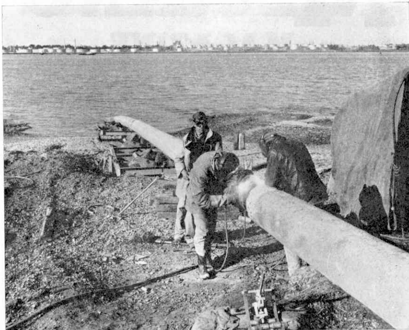
Welding two 1,100 feet sections of pipe together during the laying of a pipeline (from the Esso Refinery at Fawley to a distribution depot near London Airport) across Southampton Water. As the end of each section reached the water's edge it was welded to a following section until a continuous pipe crossed the 6,500 feet between high water levels on each bank. The lines were hauled across by a powerful winch on the Fawley shore and laid in a dredged trench which, after back-filling, ensured that they were buried at least eleven feet below the sea bed.
