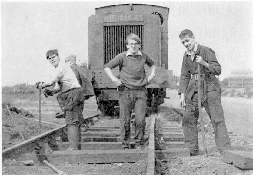
"Restoring and maintaining the permanent way . . . has been hard but rewarding work", says the author of this article. Our picture shows enthusiasts busily employed on the arduous task of platelaying.
