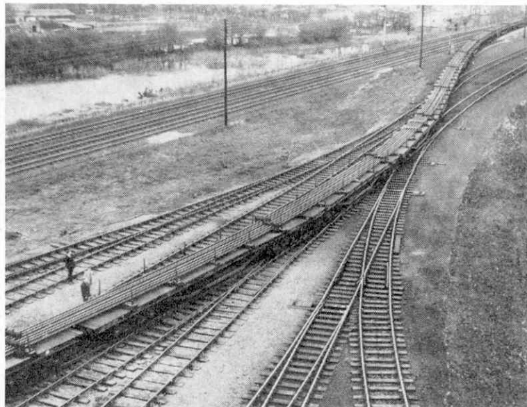
A trainload of nearly a mile of continuous welded rails leaving the Materials Depot at Chesterton
