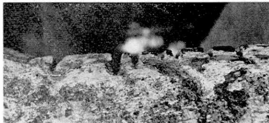
A cast-iron rubbing strip on the corner of a stone canal bridge deeply scored by the action of countless tow-ropes over the years.
