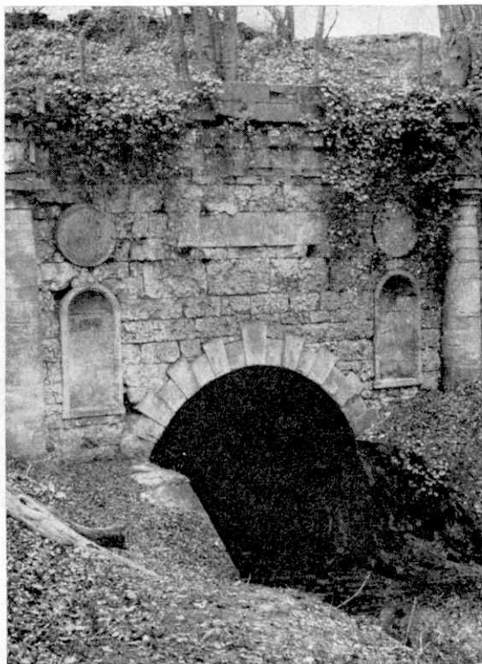
An all too familiar sight on the canals of today. This tunnel, now unused, is falling into decay.
