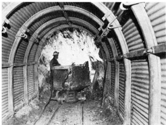
An underground gallery in an Asbestos Mine, showing the use of yieldable arches replacing the solid beam type of roof support.
